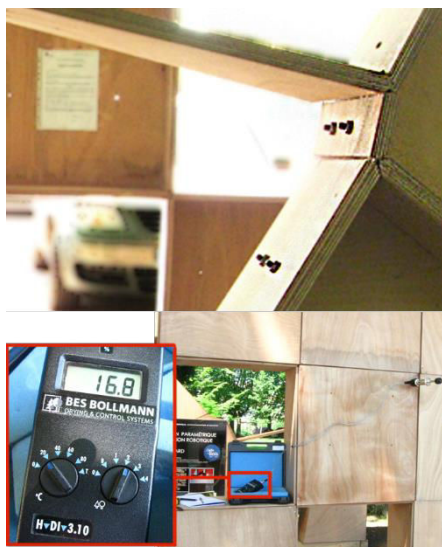
Figure 187. Top: Visual inspection and gap measurement showed no dimensional changes in items exposed to open-weather conditions. Bottom: Moisture measurement on rain-exposed cells.
