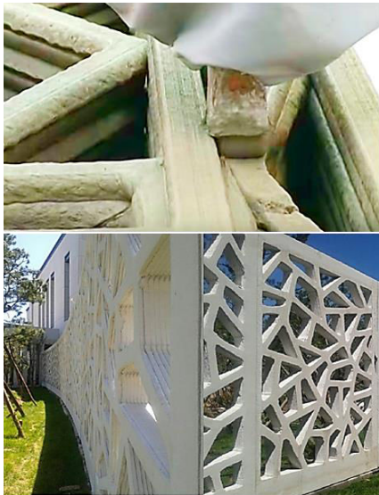
Figure 106. Full-scale house additive fabrication. This RM method, developed by Yingchuang New Materials (China), claims the ability to build the walls of a basic house in 24 hours. Using an approach similar to that of B. Khoshnevis, this Chinese company says to use a cementitious compound made of construction waste and cement to build walls. (New China TV, 2014). Top. Extrusion nozzle pouring layers of cementitious material. Bottom. Tessellated wall made using the aforementioned method. These walls were horizontally poured, then tilted-up for final placement. On: yhbm.com
