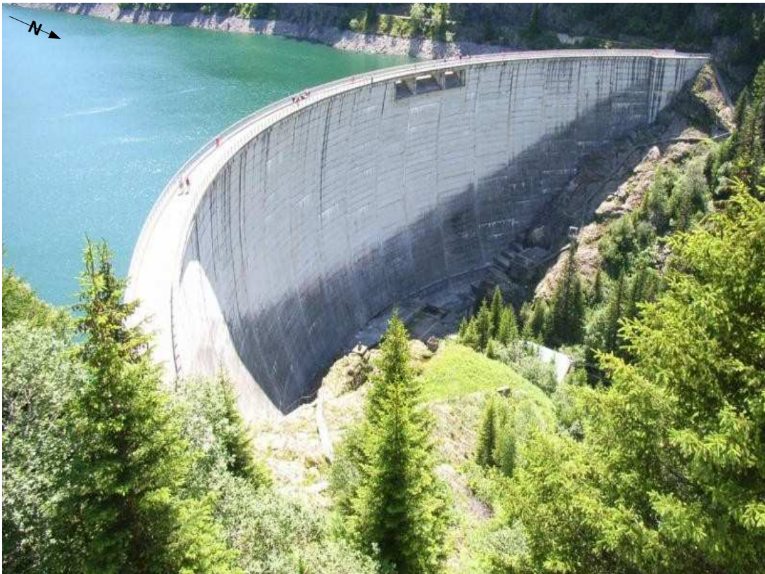
FIGURE 2.6: Double curvature, 69 m high and 250 m long arch dam in Saint Guérin.
