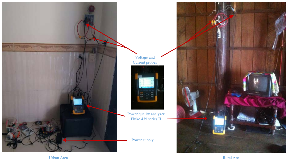
Figure IV-B-1: Set-Up of load profile measurements (Urban-left, Rural-right) by using Power Quality Analyzer-Fluke 435 series II
