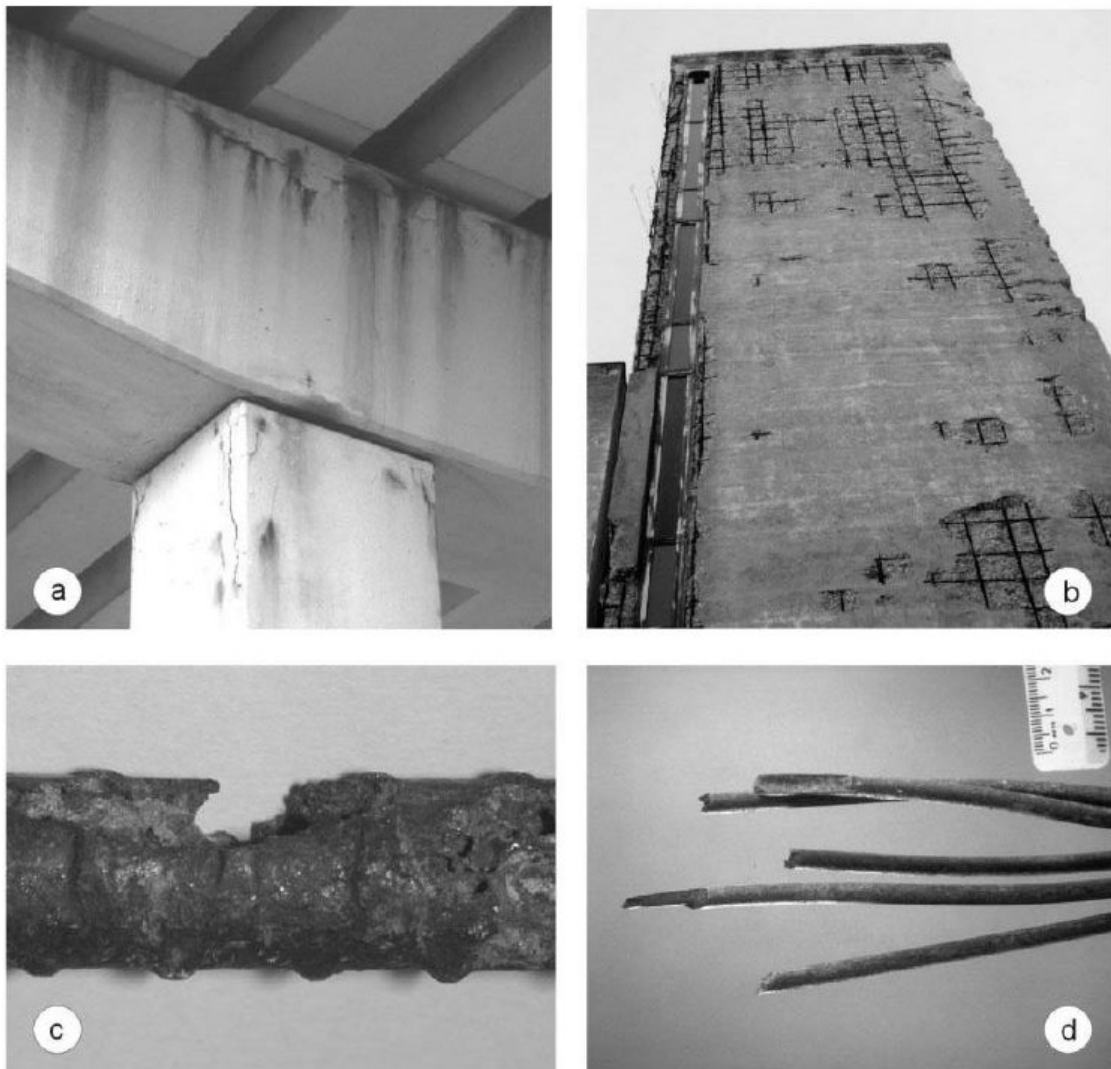
Figure 1.4: Examples of some consequences of corrosion of steel in concrete (a) cracking of column and cross beam; (b) spalling and delamination of concrete; (c) pitting corrosion causing cross section reduction; (d) brittle fracture of prestressing tendons due to hydrogen embrittlement (Bertolini et al.
