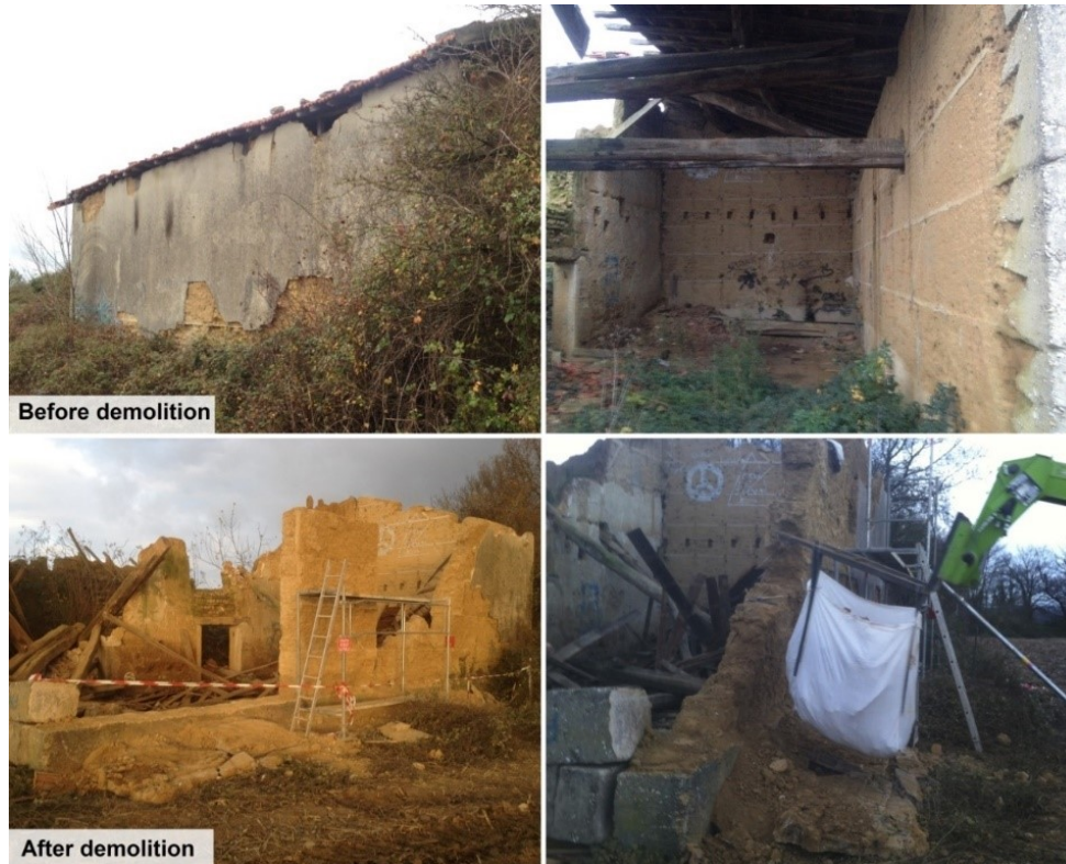
Figure 2.6 Rammed earth soil origin: farmhouse before and during the demolition, (Photo: N. Meunier)
