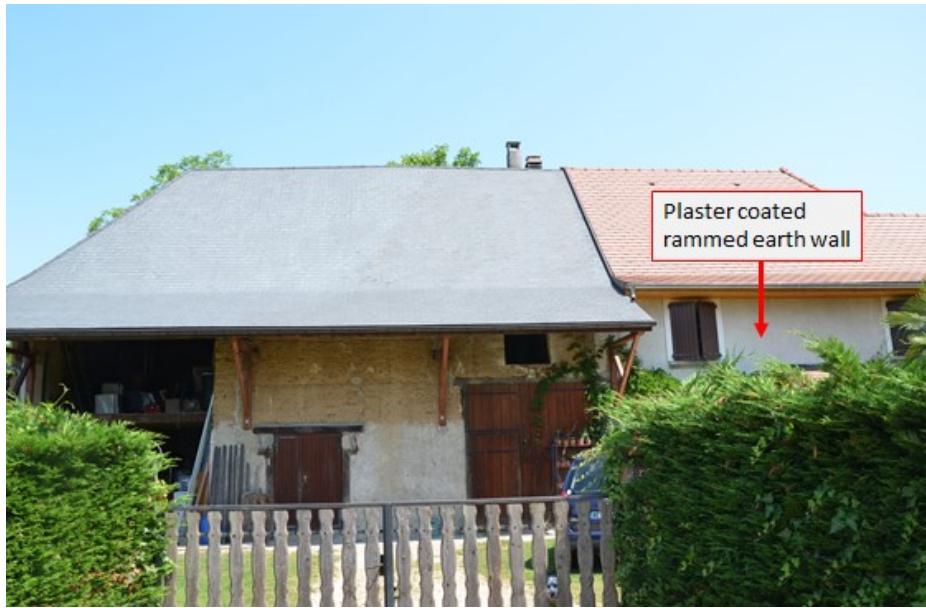
Figure 1.17 Renovation of a part of rammed earth house in “Pont de beaux voisins”, Rhône-Alpes, France
