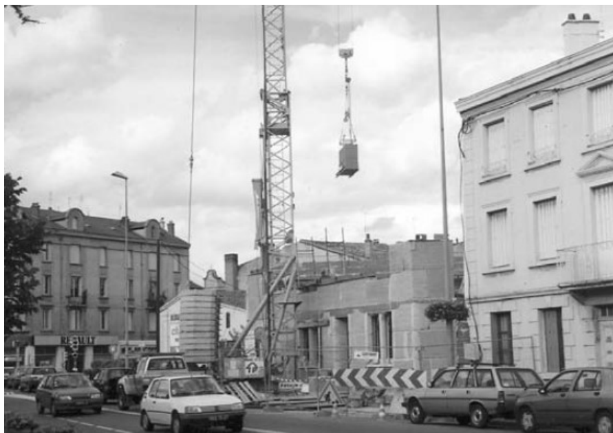
Figure 1.21 Pre-fabricated walls being craned into position during construction at Montbrison, Loire (Photo: N. Meunier, 1995)
