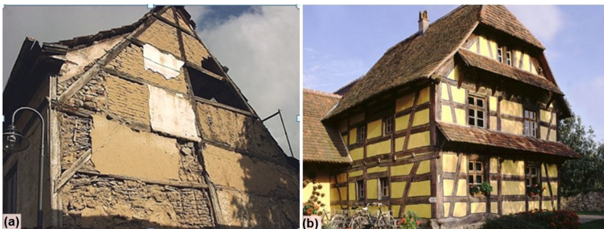
Figure 1.2 (a) Building in the central German city of Bad Langensalza made of wattle and daub (Photo: Sebastian Wallroth); (b) House in France, Alsace (Photo: Auroville Earth institute)
