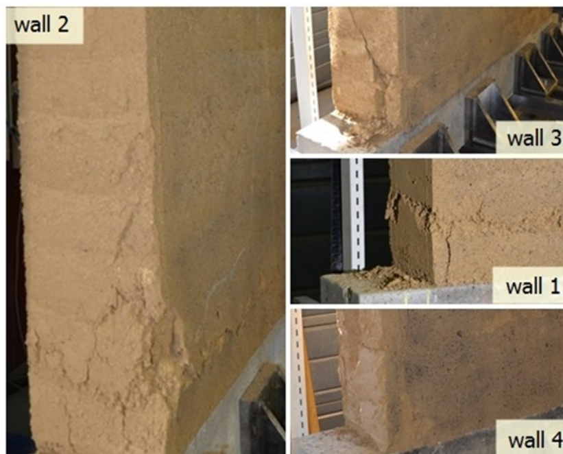
Figure 3.31 Crushing on the left side for different walls during the test
