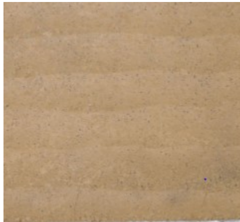
Figure 1.11 Visible compacted layers with different thickness of a rammed earth wall constructed in the LOCIE laboratory
