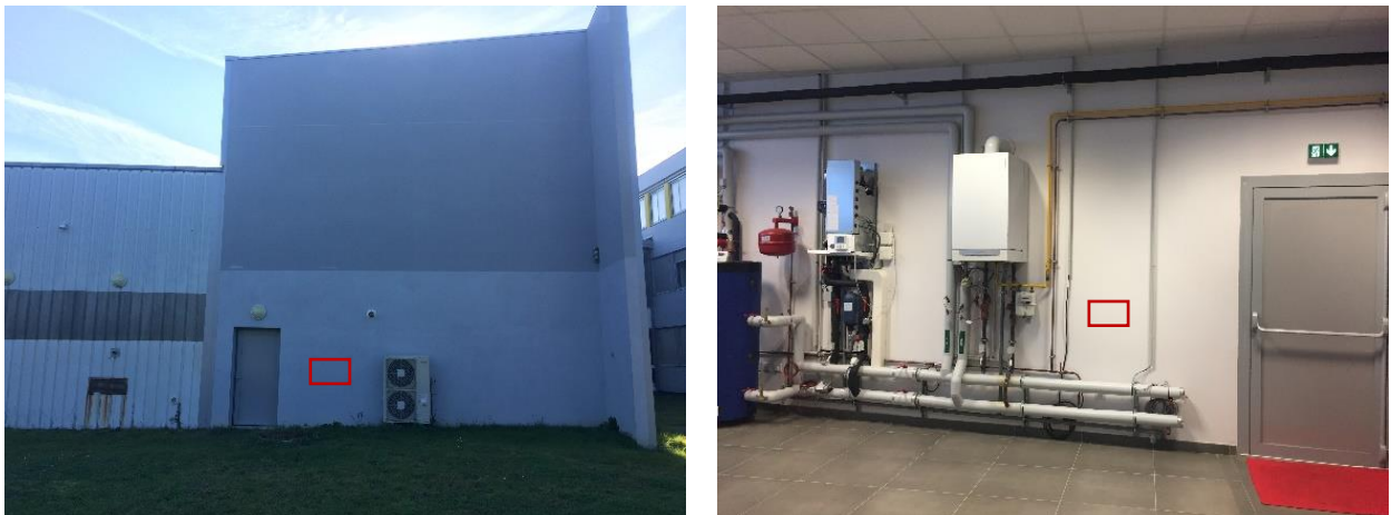
Fig. 2-22 The exterior wall of building that to be tested: outdoor (left) and indoor (right).
