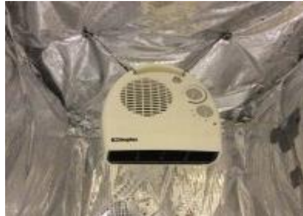
Fig. 2-19 Heater installed inside the wall box
