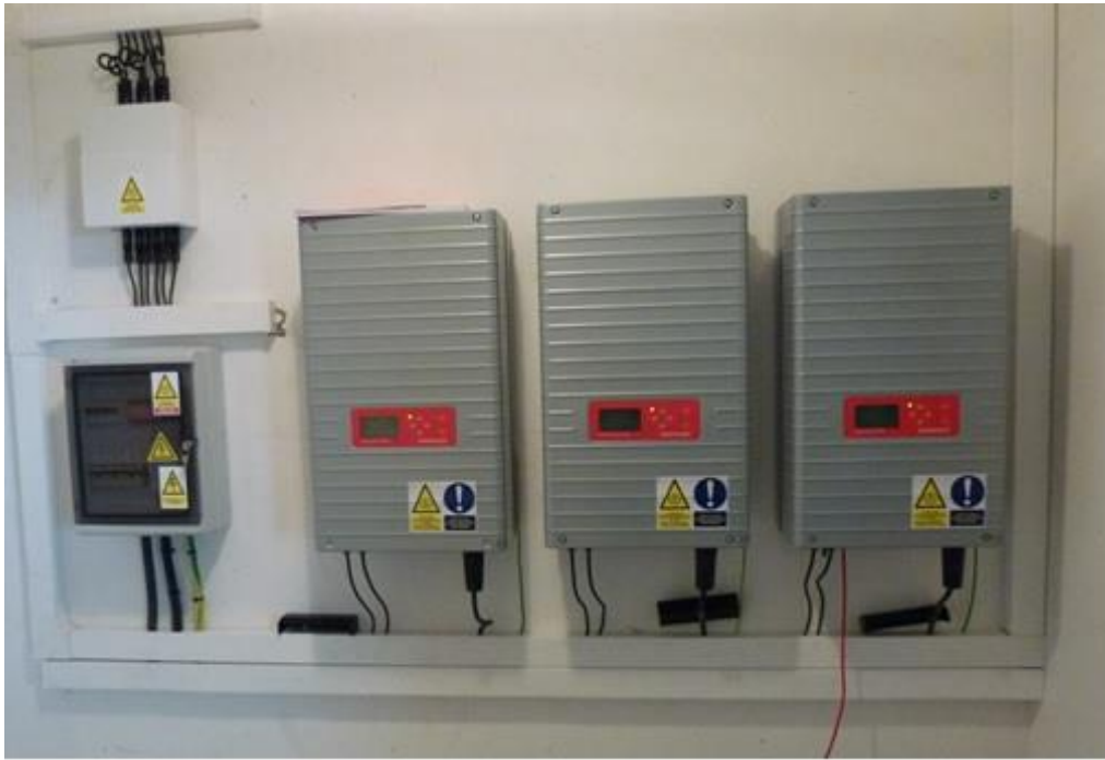
Figure V-11 Three solar PV inverters with 0.6 kWh daily output for each.
