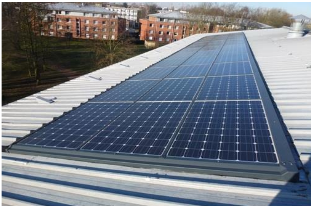
Figure V-10 PV panels installed on the roof of the student residence of Centrale de Lille.
