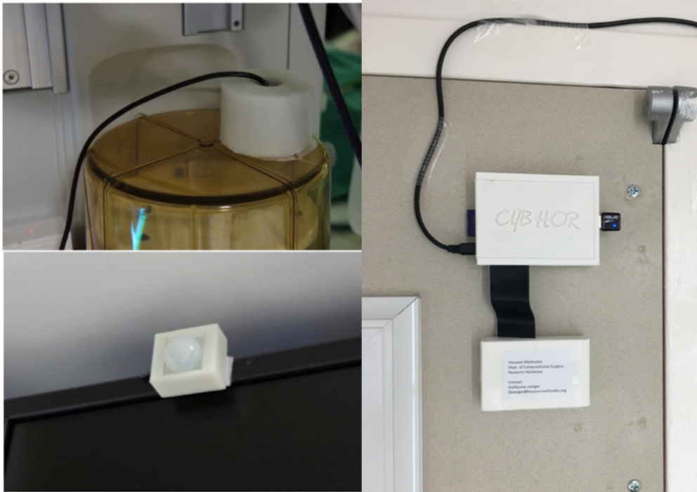
FIGURE 2.5: Final array of sensors installed in 5 ORs of the hospital. On the top left you can see the camera placed on top of the bellow of the anesthesia machine with Velcro. On the bottom left there is the IR motion sensor placed in a corner of the room. Finally, placed on the door you can see the 9-DOF sensor connected to the raspberry pi with its Wi-Fi dongle.
