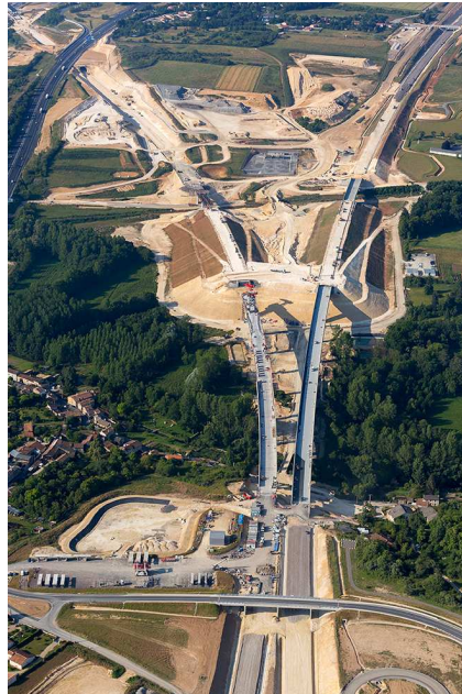
Figure 2.3: Aerial view of part of a stretch of the SEA line; source: Vinci Construction Terrassement
