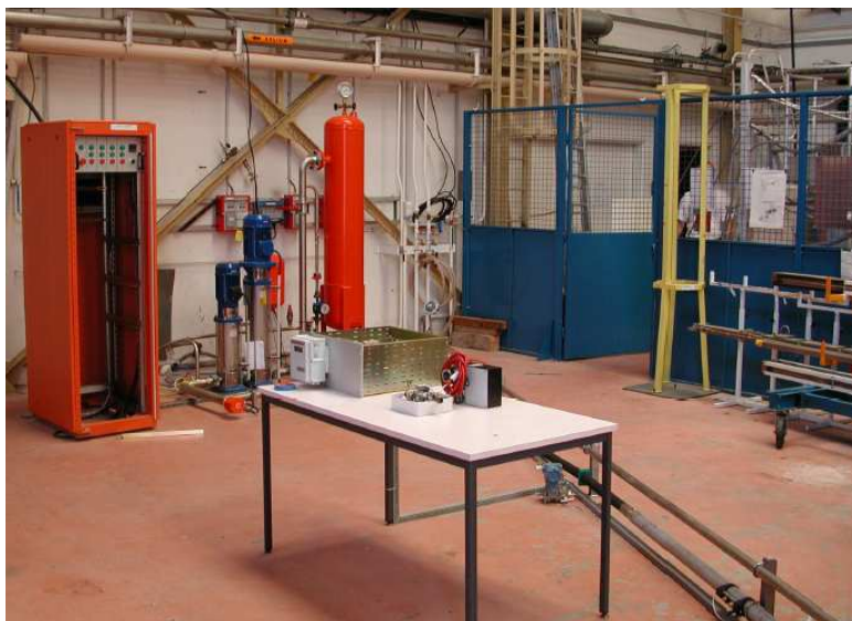
Figure A-6: HECOL facility
