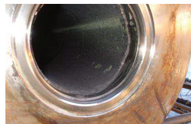
Figure 4: Sulphide scale in topsides flowline
