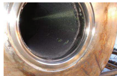
Figure 4: Sulphide scale in topsides flowline
