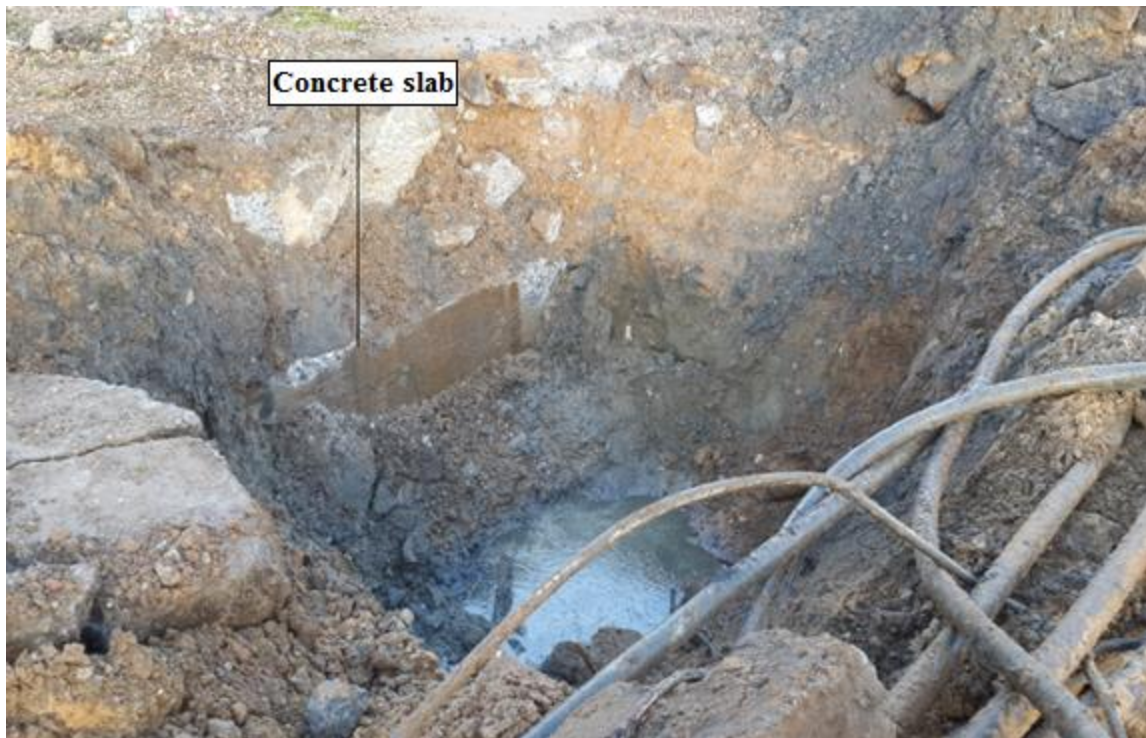
Figure 7.8: An excavation done along profile P5 showing a buried concrete slab at a depth of around 1m.
