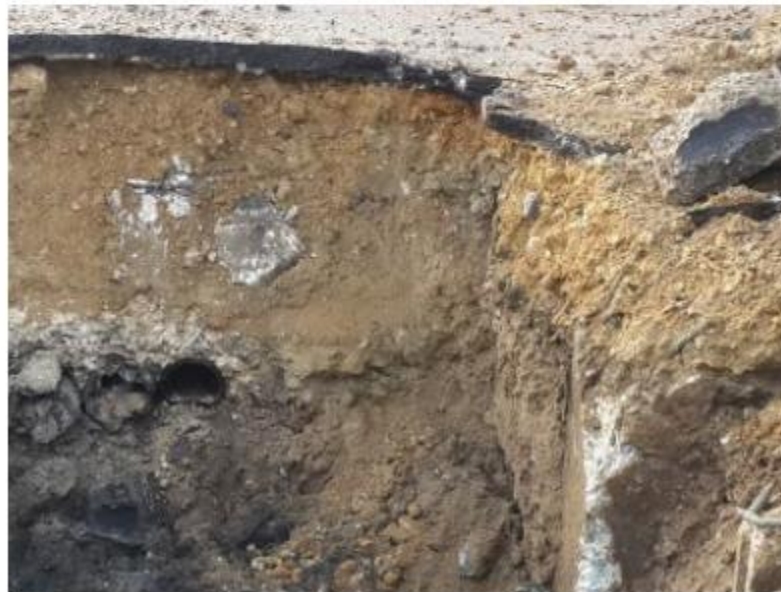
Figure 7.9: Excavations done along profile P1 showing buried water and oil supply pipes. The narrow hyperbolas in the GPR profiles represent the water supply pipes while the wide hyperbolas represent the oil pipes.
