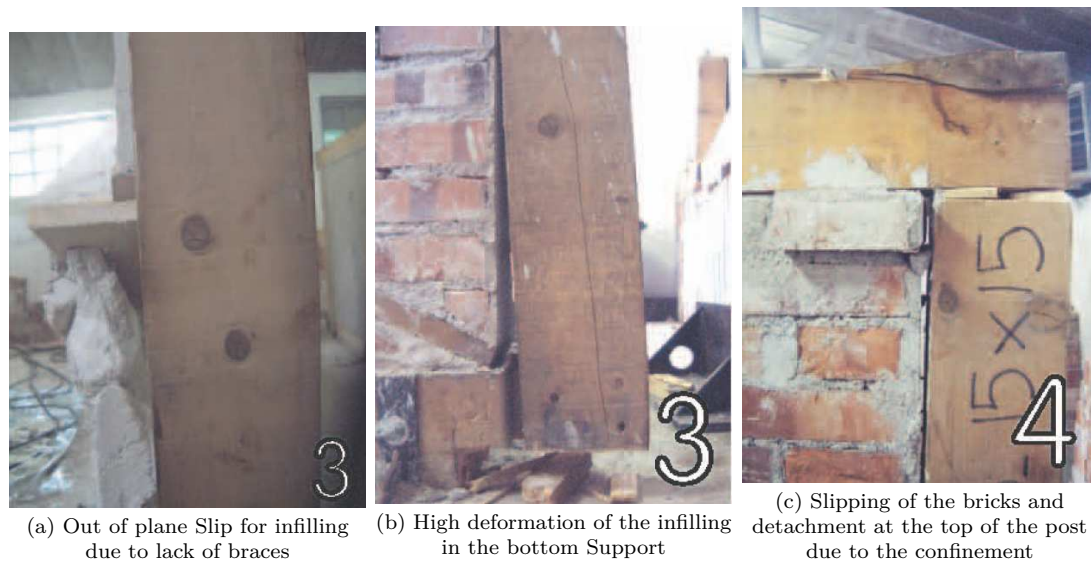
Fig. 2.27: Modes of Failure of Maso Wall by Ceccotti et al. [27], [135]
