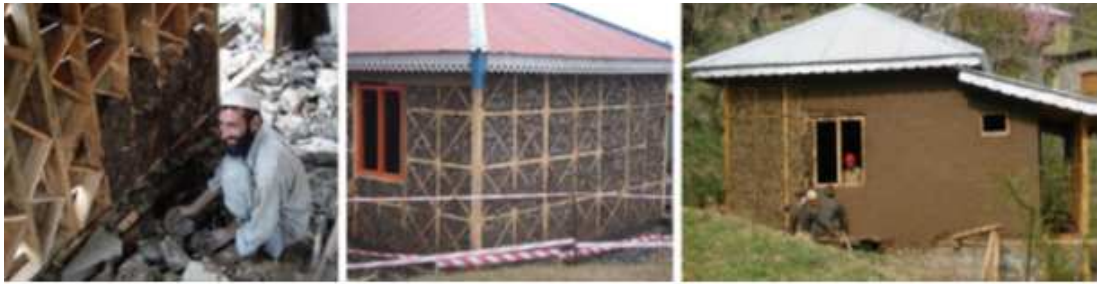
Fig. 2.6: Sample of Dhajji Dewari system in the north of Pakistan, Ahmad et al. [4].
