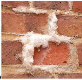
(a) Efflorescence (whiskers)
