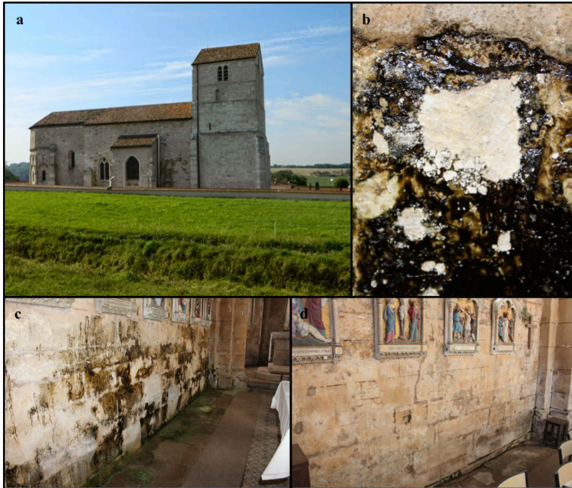
Fig. 1. Illustration of Vicherey church (a) and its biodeterioration (b) due to biofilm proliferation. Wall with southern exposure and floor of the church were affected by microalgae and cyanobacteria (c), while north exposed wall was less invaded (d).
