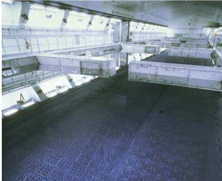
Figure 1.22 – Wet storage: CLAB pool for wet storage in Sweden [50].
