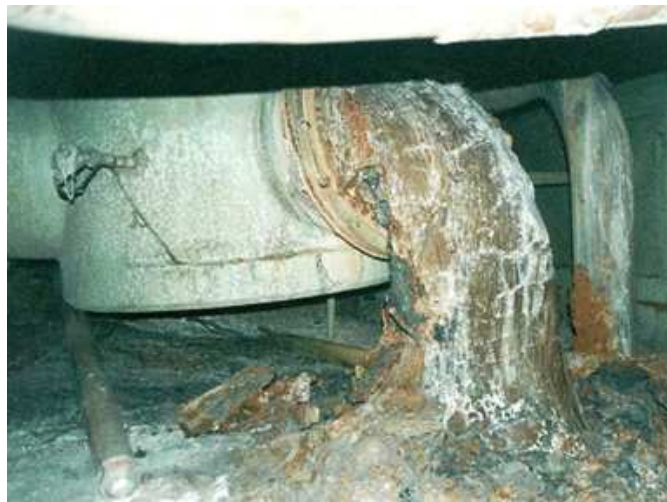
Figure 1.29 – : Solidified LFCM flowing out of the 4th steam-distribution valve in Room number 210/7.
