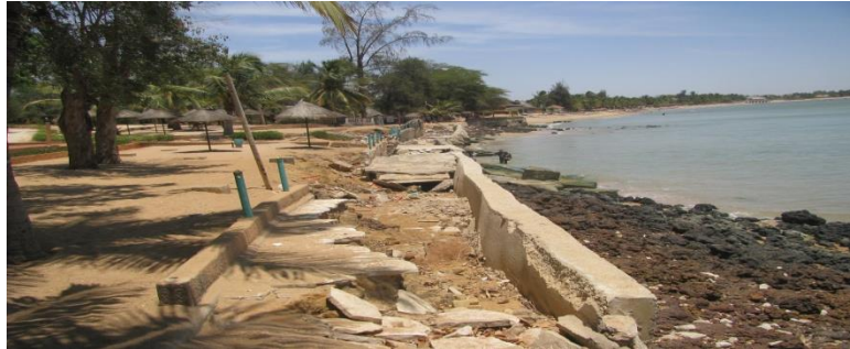
Photo 19 : Photo savana (rupture mur de protection)
