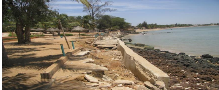
Photo 19 : Photo savana (rupture mur de protection)
