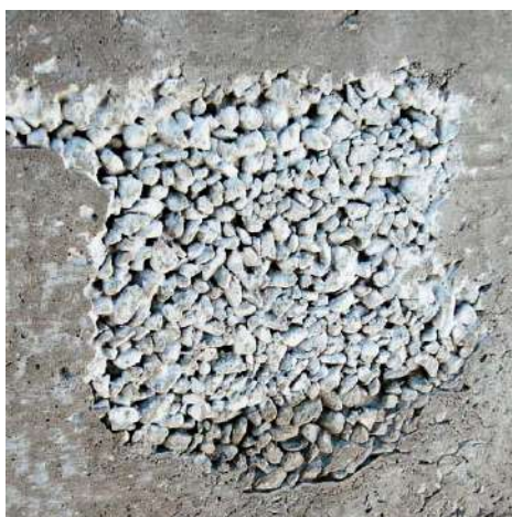
FIGURE C.3 – nid de gravier (Blasting, 2018)
