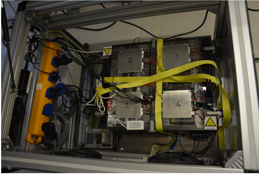
Figure 4.5: Inside the rack: the enclosure is wrapped in ropes and fixed on a aluminum plate.
