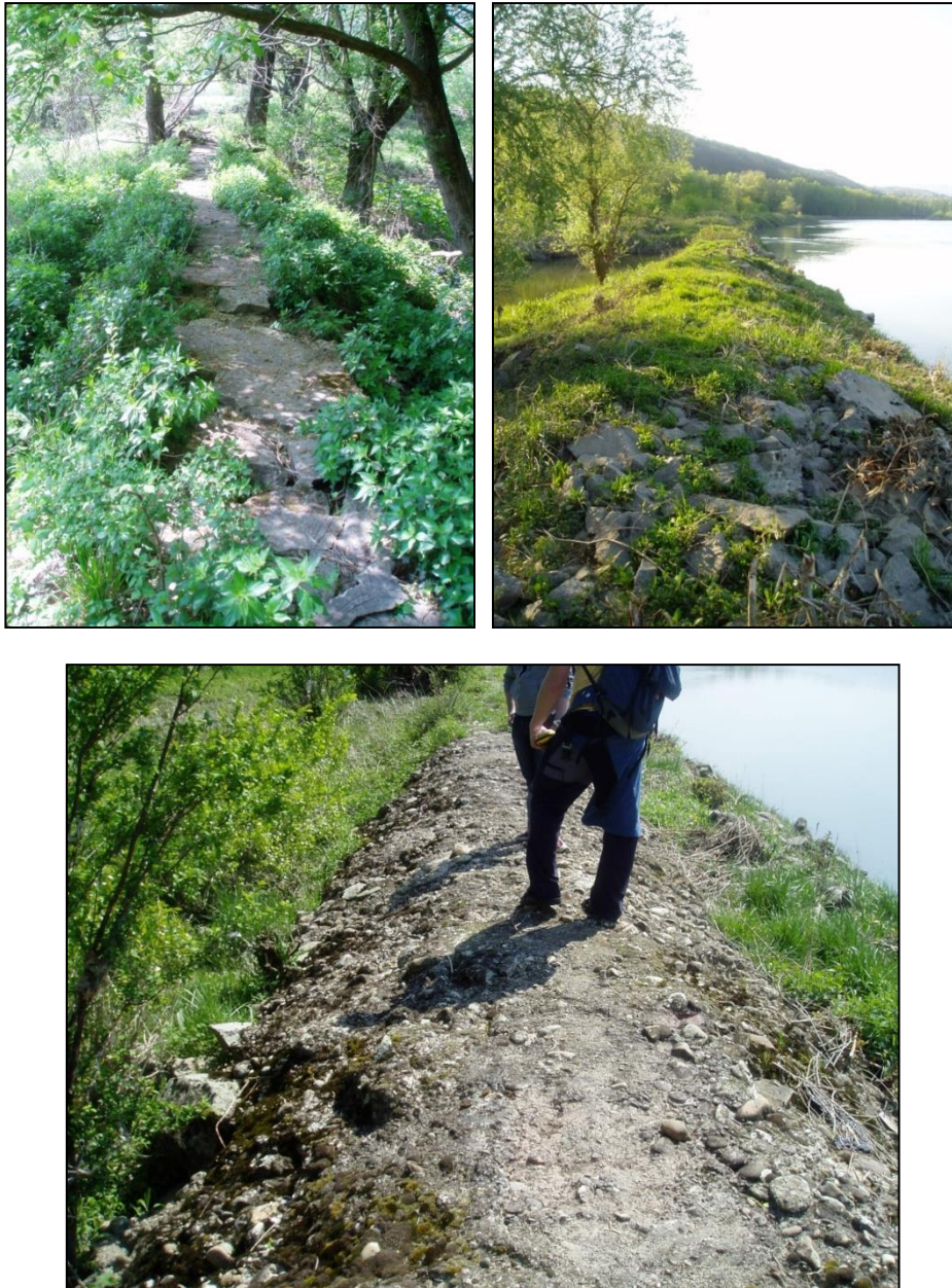
Figure A-I-2: Examples of different dike construction materials with potentially different seepage potential.
