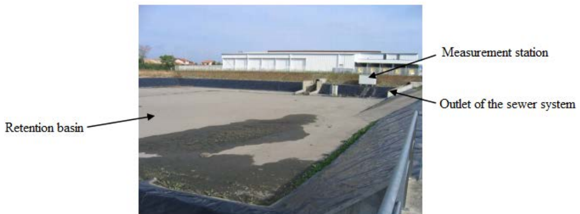
Figure 3. Photo of the measurement station installed at the outlet of the stormwater system (inlet of the retention basin) (source: Métadier, 2011).
