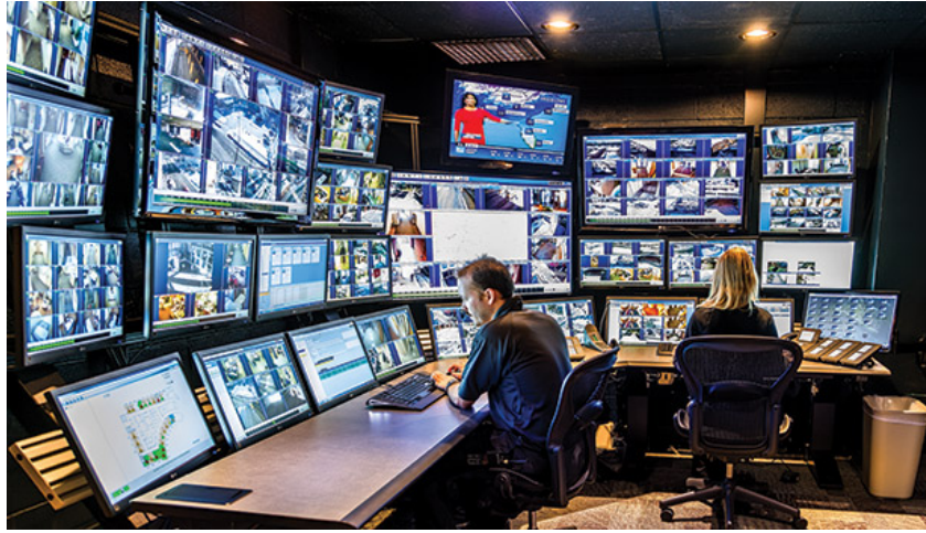
Figure 1.2: A video surveillance system control room.
