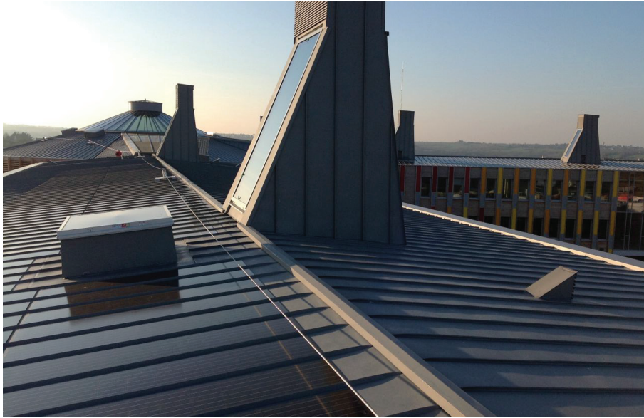
Fig. 1.4 Solar chimneys on the roof of public building in Côtes d'Armor, Brittany, France. Credit: Agence Nicolas Michelin & associés
