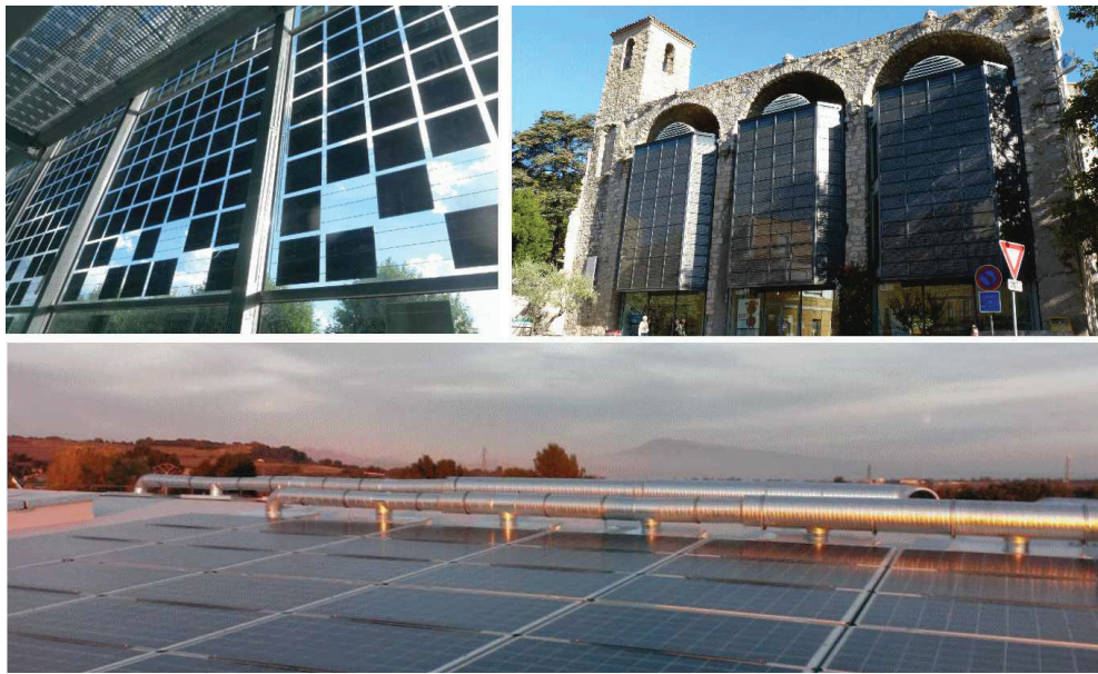
Fig. 1.6 BIPV systems, (top left), integrated solar cells on the outer skin of a double skin façade at the Schneider electric building, Grenoble, France, (top right), similar system at the tourism office of Alès, Cévennes, France, (bottom) assisted hybrid thermal-photovoltaic designed with EPC Solaire in the context of the ADEME project Horizon PV
