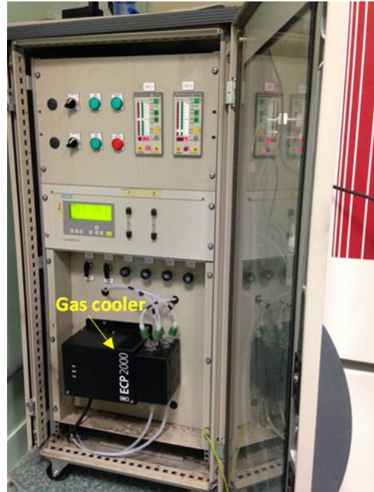
Figure 2-19: Siemens cabinet of CO 2 analysis and control
