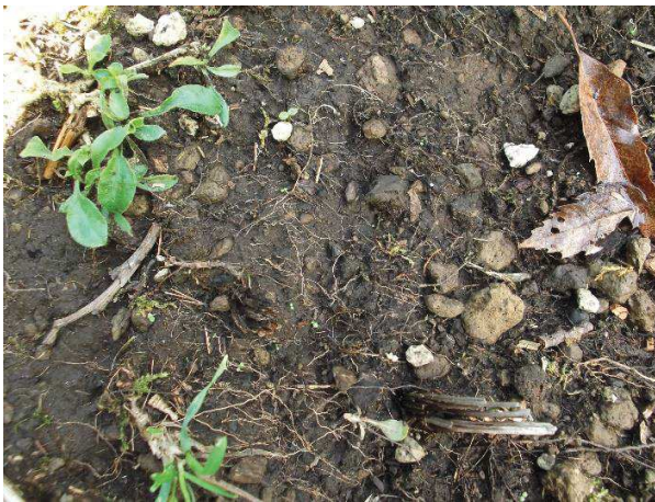
Figure 41 – Soil erosion exposing roots.
