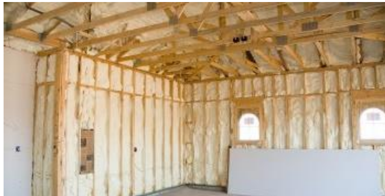
Fig. 0.5 – Plastic foam insulation of buildings.
