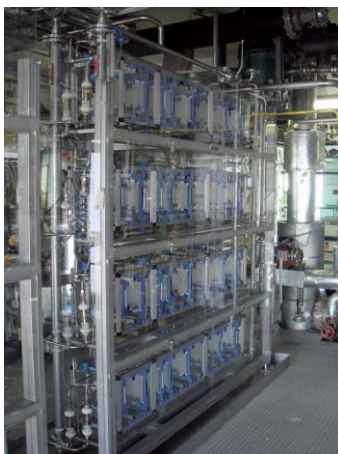
Figure 14 Production bank with four identical reactors and distribution 45
