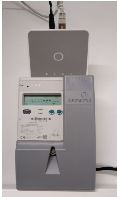
Figure 4.9 – Kamstrup Smart meter
