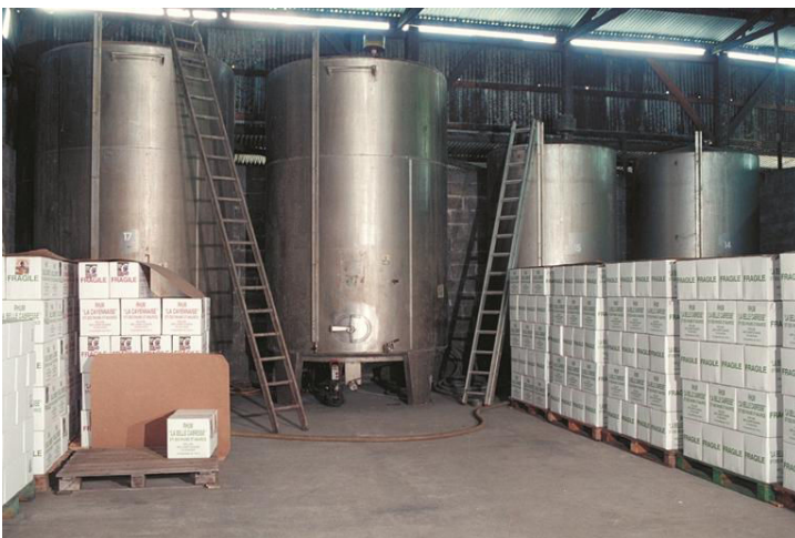
Figure 13 : cuves de stockage
