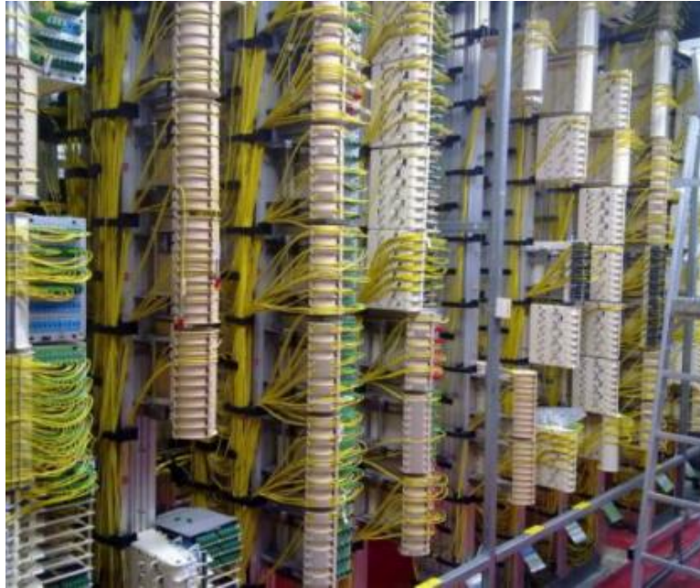
Figure 236 : Example of a distribution cabinet
