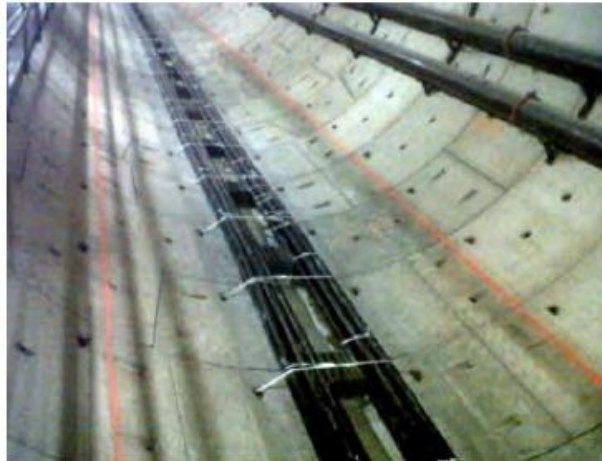
Figure 201 : The High Voltage Electrical network integrated in the metro infrastructure. This picture shows an example of mutualization between a metro tunnel and an energy tunnel.
