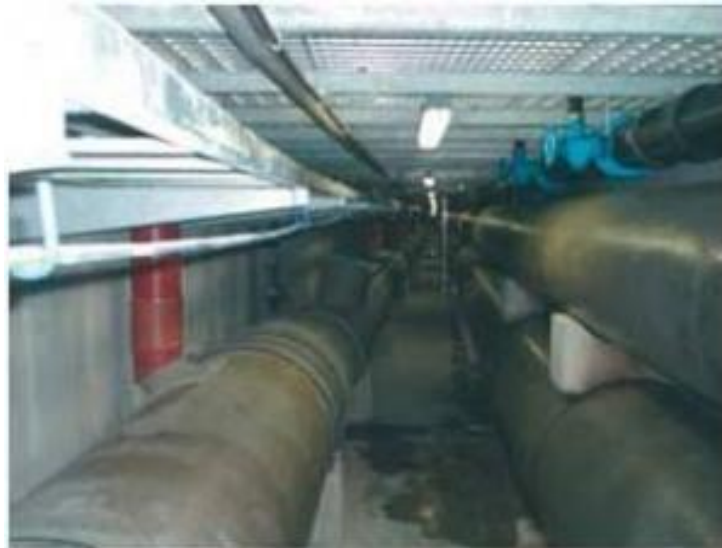
Figure 6: Utility Gallery, Geneva, Switzerland. The utility gallery is a multifunctional structure which welcomes all types of urban utilities (electricity, water, optical fiber, gas).
