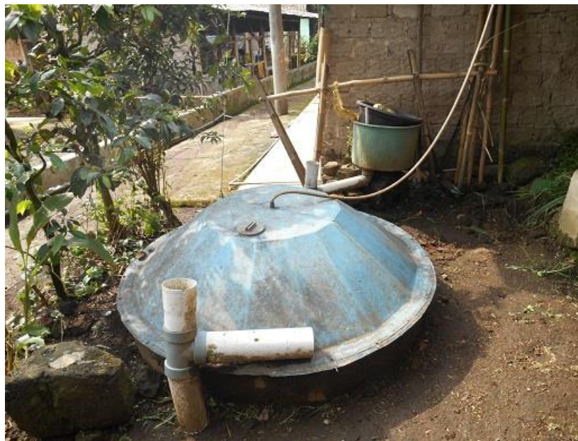
Figure 30 Biogas installation in the farm
