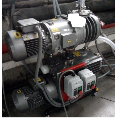
FIGURE 7.2: The roughing pump is a combination of an E2M80 rotary pump with an EH250 mechanical booster (both from Edwards Vacuum Ltd), yielding a pumping speed of 274 \text{ m}^3/\text{h} .
