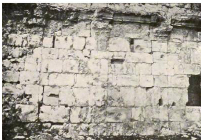
Al- Ruṣāfa: gates north gate_ east interior wall of the propugnaculum (Musil Alois)
