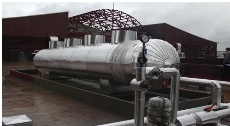
Figure 0-19: Storage tank implemented in a real solar cooling installation at the University of Sevilla (Spain) [58]
