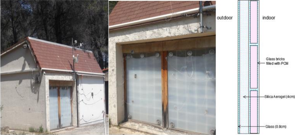
Figure 4-2: TIM-PCM wall from the outside and Schematic of the TIM-PCM wall composition
