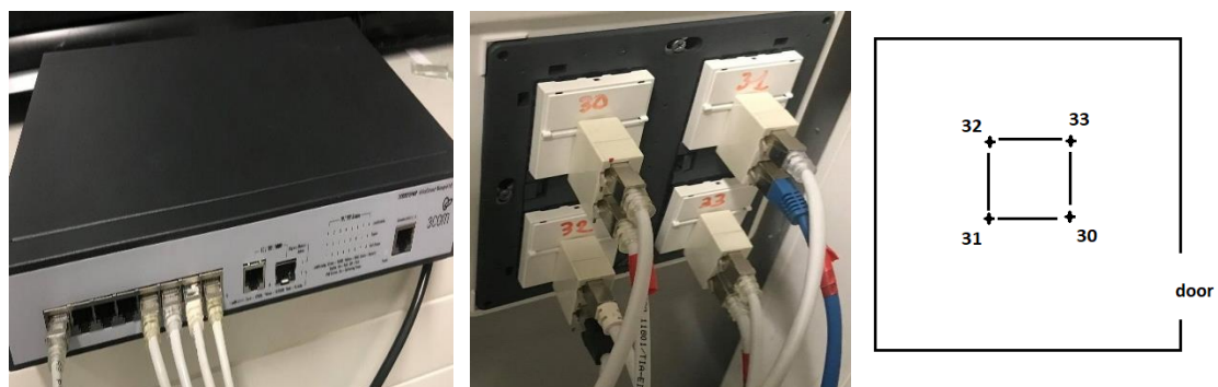
Figure 3.31. Switch connection and positions of receivers in the room with their numbering
