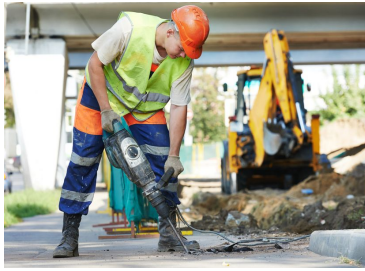
(a) In public works, painful working posture and discomfort caused by noise and vibrations of tools.
