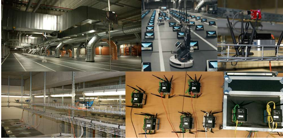
Figure B.6: Hardware employed in the testbed and the scenario where it is deployed.
