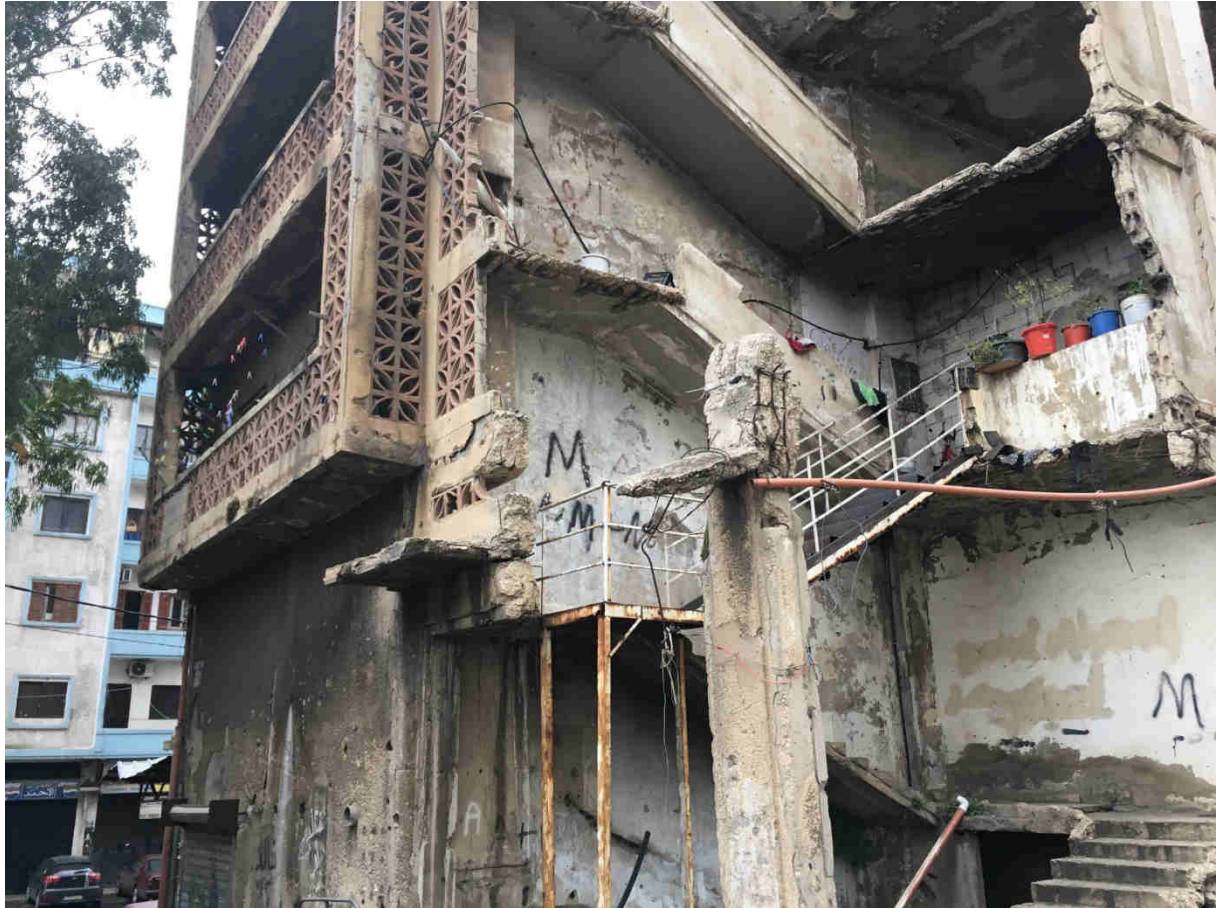
Figure 7-2: A Syrian refugee family lives in a building with degrading structure Tebbeneh. October 2018
