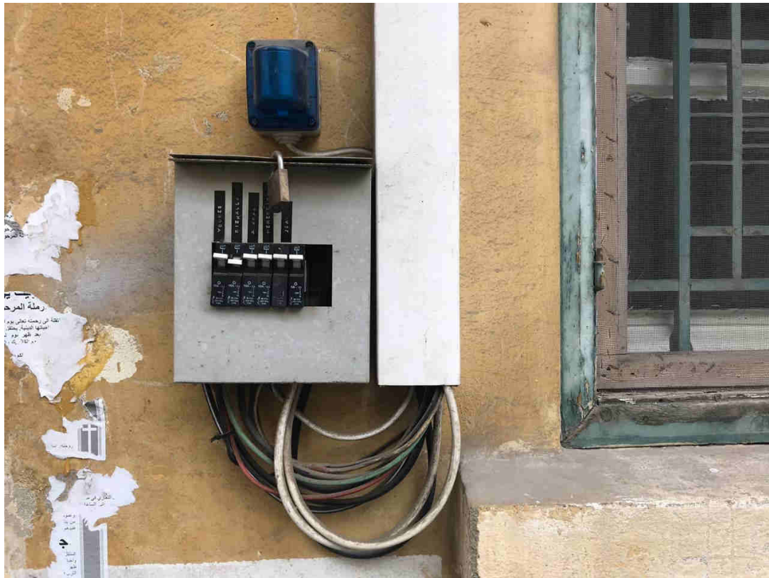
Figure 3-13: Private Generator signals
