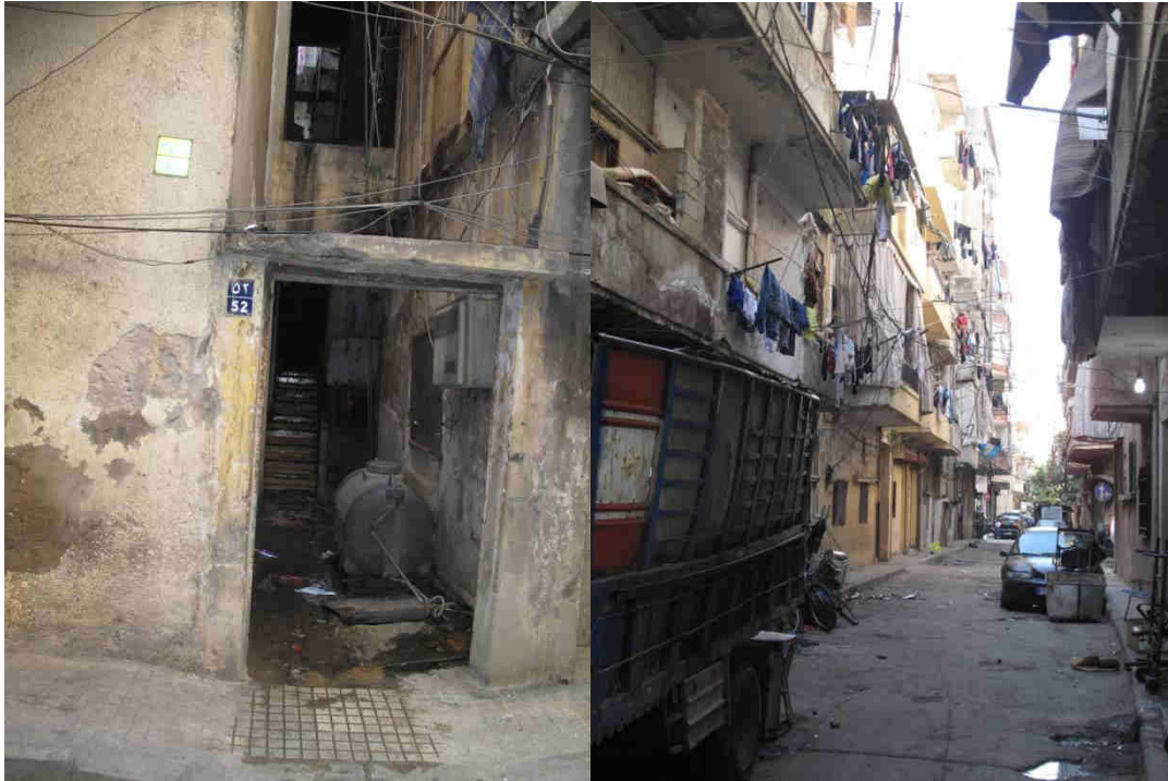
Figure 5-21: Urban deterioration in EL-Nab'a
