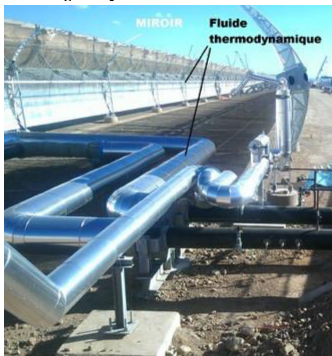
Figure 2 photo de la centrale Noor 1
