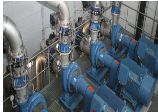
(b) Station de Pompage
