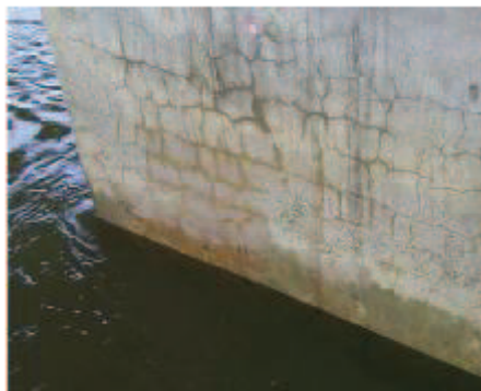
Figure 5.13 – Example of bridge pier presenting cracks induced by delayed ettringite formation - [Godart and L. Divet 2013]
