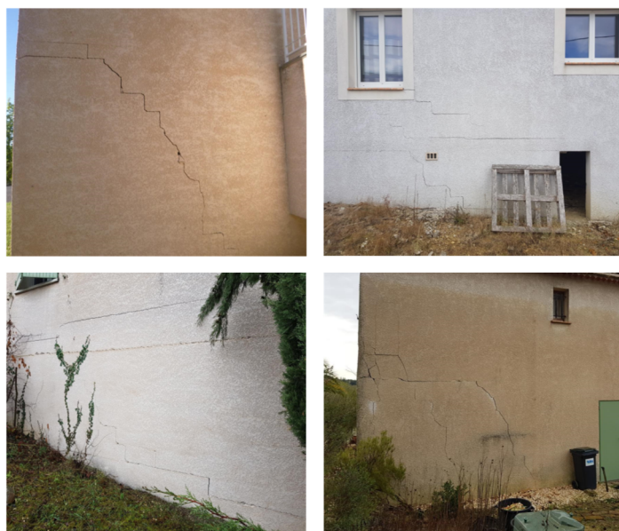
Figure 1.2 - Some examples of cracked residential buildings due to shrink-swell of clays.
