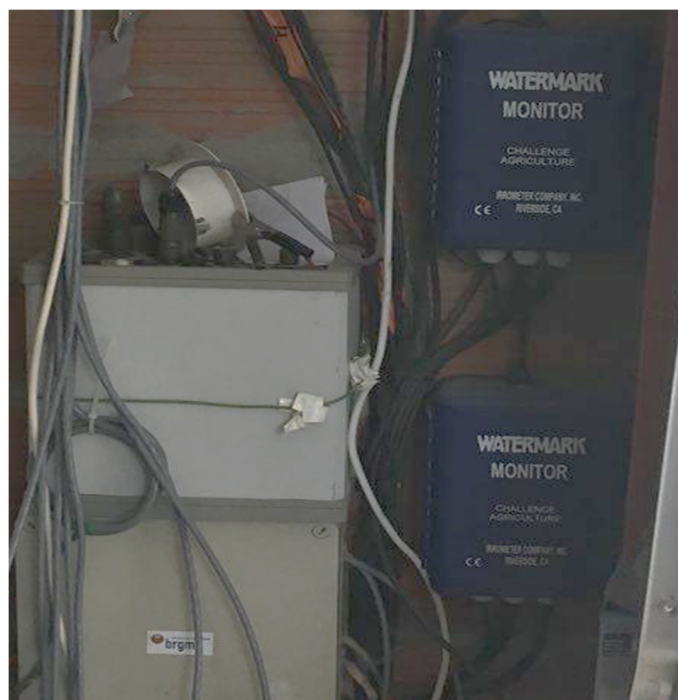
Figure 3.7 - Different data loggers used in the monitoring operations
