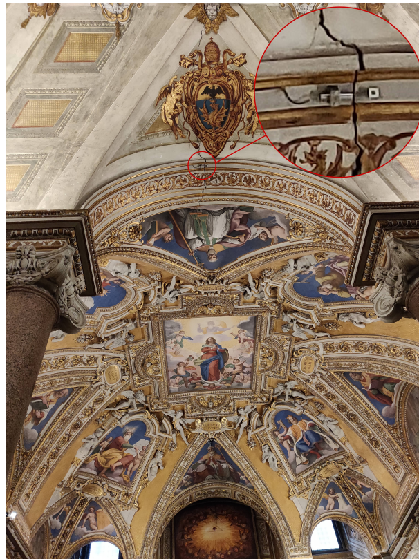
Figure 2: Monitoring of crack opening at Basilica Papale di Santa Maria Maggiore (Photo credit: T. Heitz)
