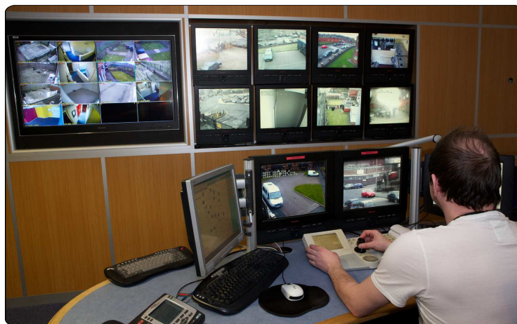
Figure 2.2 – Classical monitoring room.
