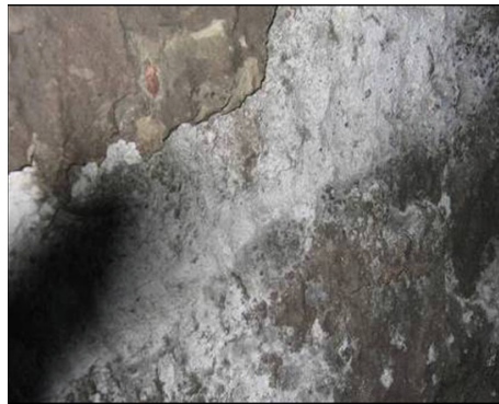
Figure 1.2 – Surface concrete spalling exposed to sulfate-rich environment [4].
