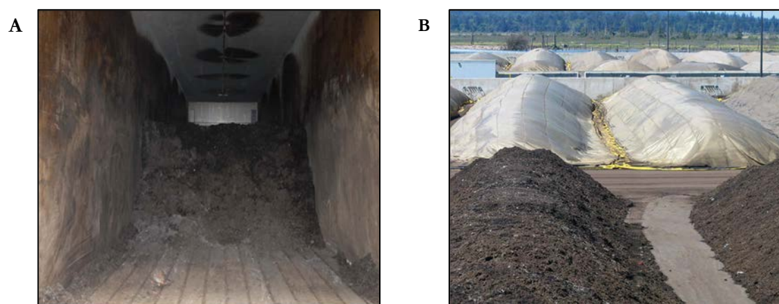
Fig. 10. Concrete tunnel for in-vessel composting ( A ) aerated static pile covered by semi-permeable membranes ( B , Gore®)
