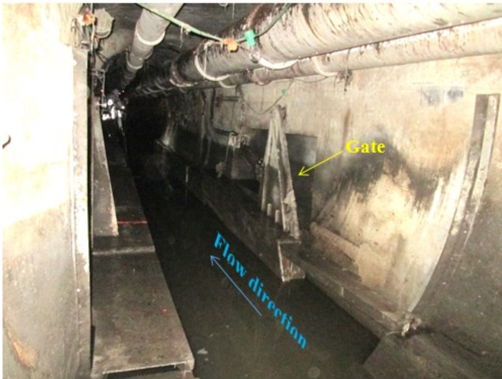
Fig. 3.5 Implemented gate being as a radial tipping gate with weir function.
