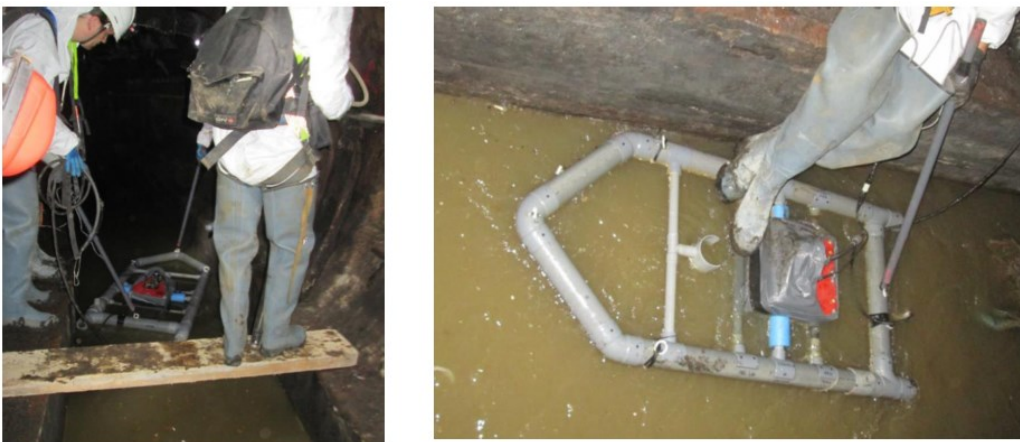
Fig. 3.10 The bed scan apparatus developed to measure the sewer bed topography before and after the flush.
