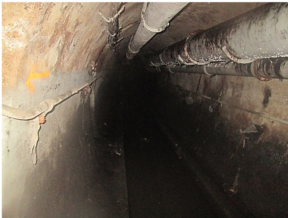
Fig. 3.3 Studied sewer channel with pipelines installed on the top of the channel.
