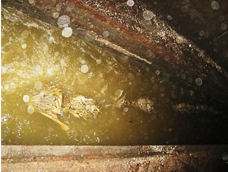
Fig. 3.8 Image of floating sewer deposits of rags/resin-type sediments through the studied channel.
